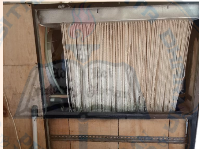
Gambar 3.8 Cooling Pad Tampak Samping
