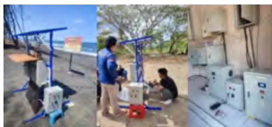
Fig. 4.2. Testing of Electrical Energy Monitoring Tools
