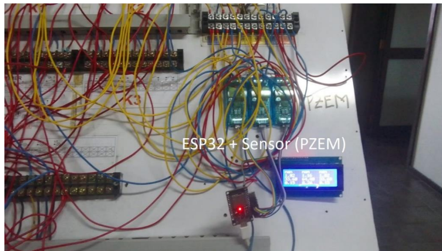
Figure 5. Installation of three PZEM-004T sensors on motor terminals with ESP32 and 20x4 LCD
